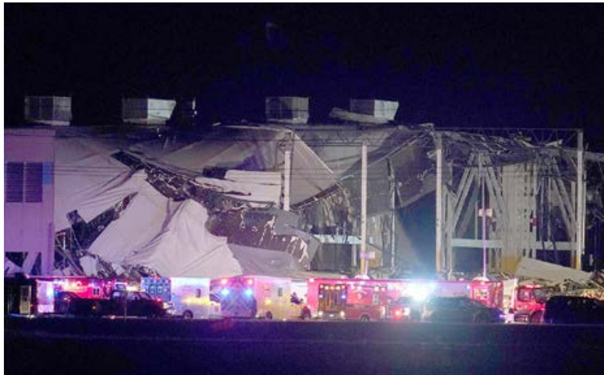
THIS AMAZON FACILITY COLLAPSED AFTER A TORNADO HIT IT IN EDWARDSVILLE, ILL.
